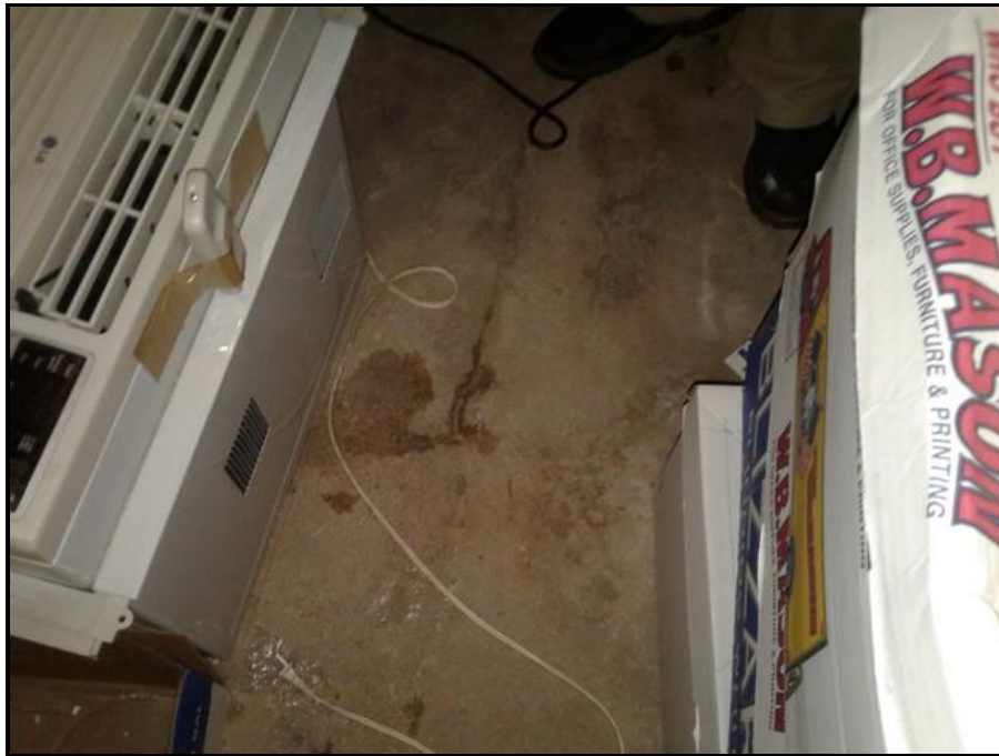
Water penetration at floor
