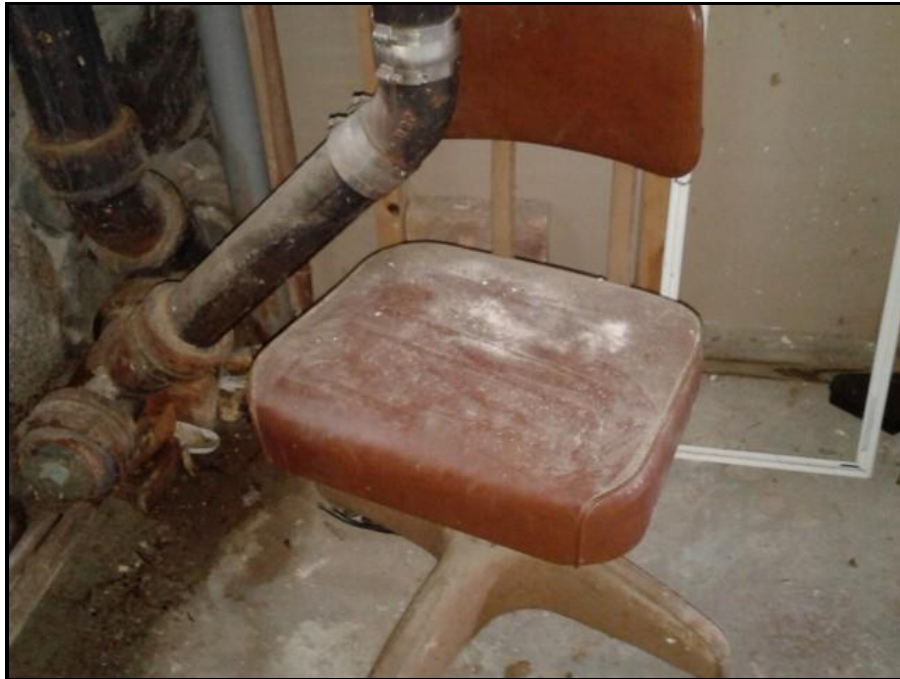
Suspect mold on stored items and debris
