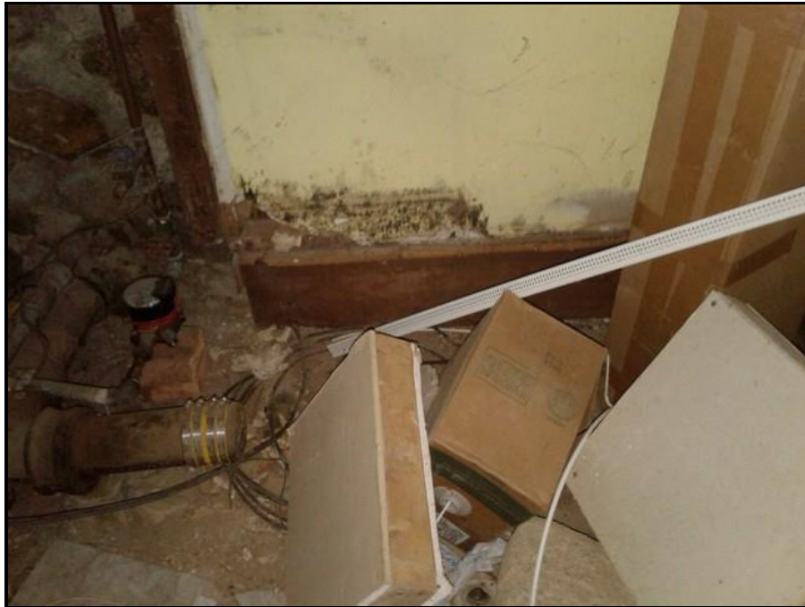
Suspect mold on sheetrock wall
