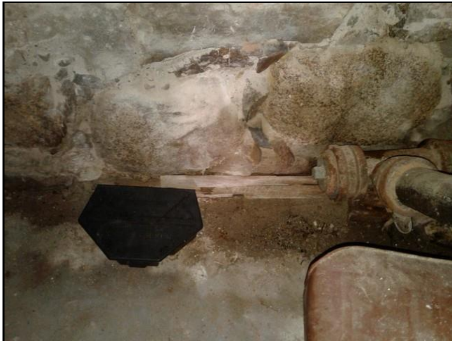
Water penetration at rear foundation
