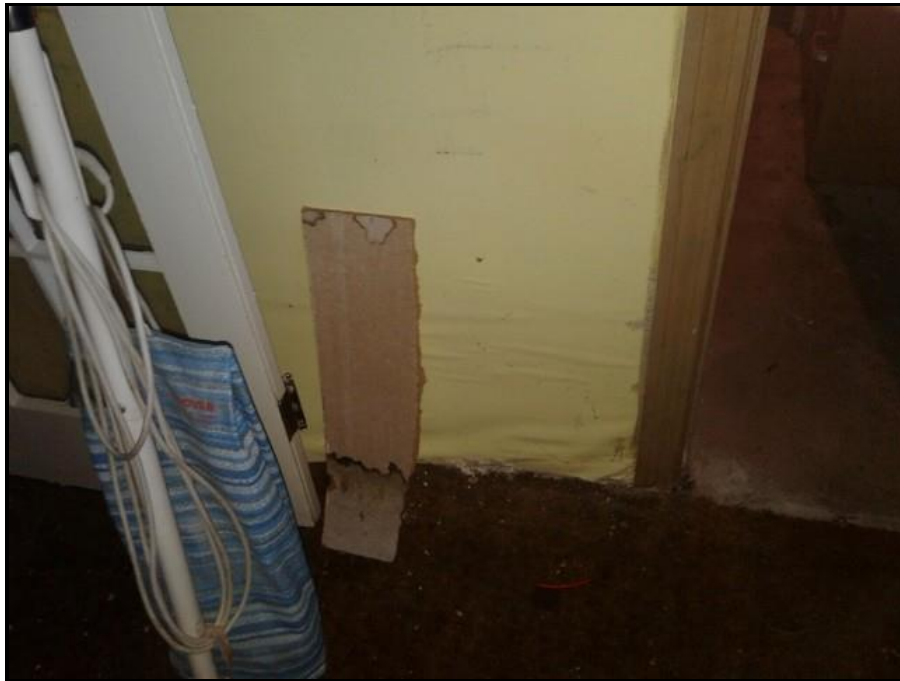
Water damage to wall
