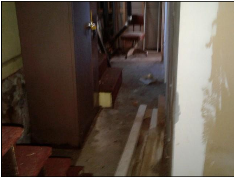
Suspect mold on stored items and debris
