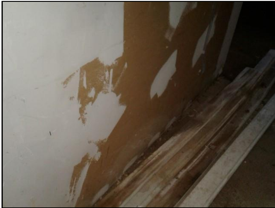
Suspect mold at rear storage area wall
