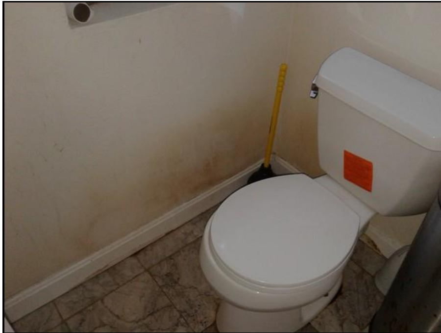
Suspect mold in bathroom
