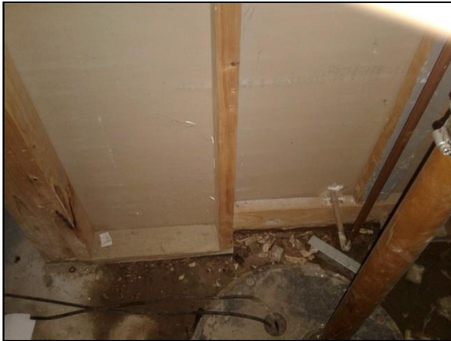
Water staining at storage area floor
