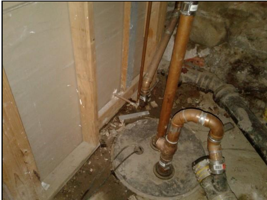
Water penetration at floor
