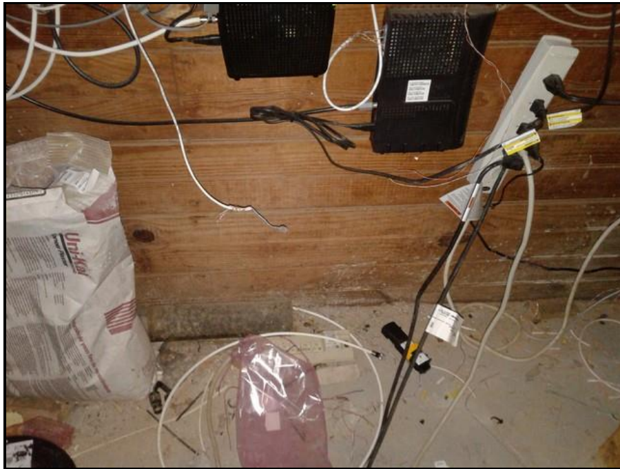
Suspect mold on wood wall
