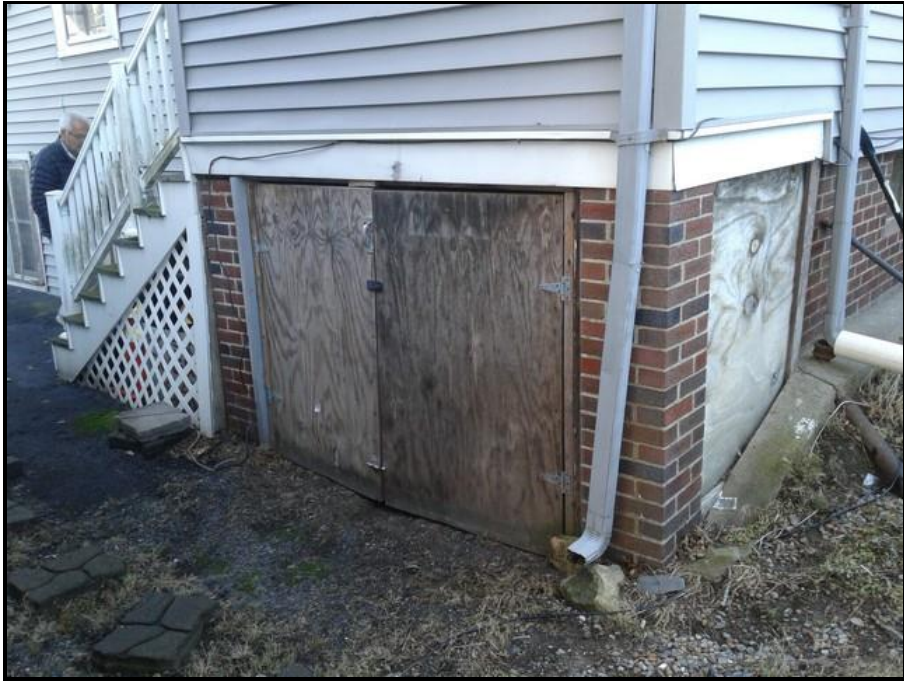
No extension at down spout
